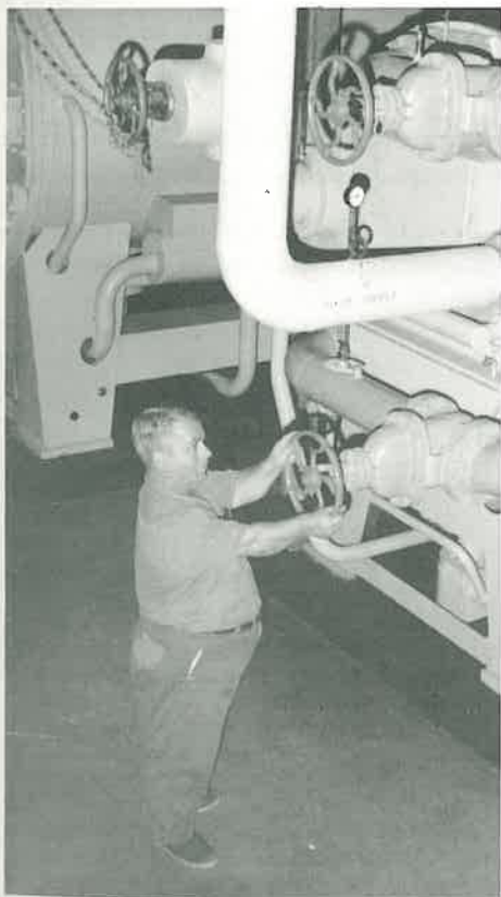
Joe Woods, known as "Shorty" because of his slightly less than 5-foot stature, adjusts water pressure in the boiler room. Some of the best housekeeping to be found anywhere is in the powerhouse, where the employees take particular pride in its neatness. Even the concrete floor is waxed.
