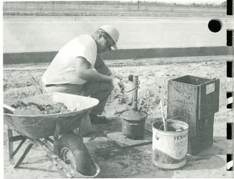
Rick Matthews worked on the job as a summer employee. Here he makes a air content test to determine the amount of air mixed with concrete. Matthews, of West Memphis, has now resumed his studies at Arkansas State University in Jonesboro.
